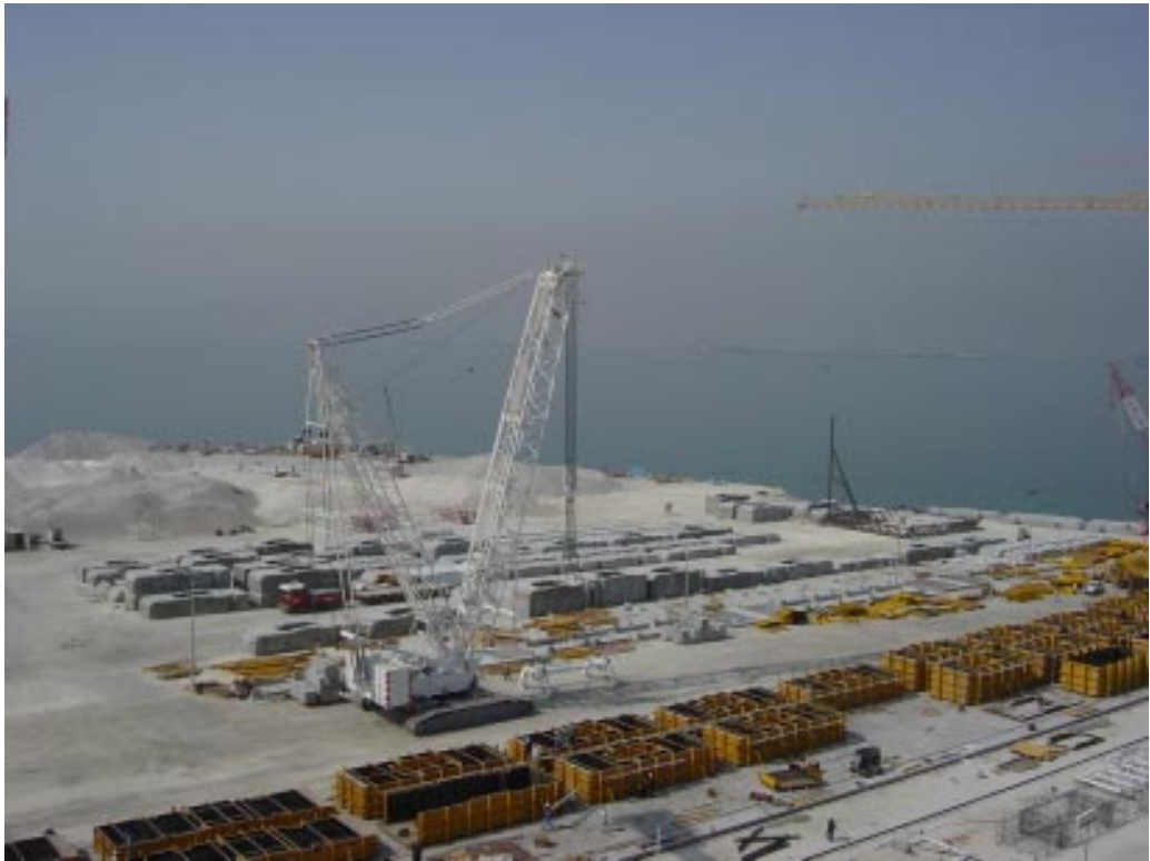
The concrete casting beds and storage area at the Shaikh Khalifa Bin Salman Port in Bahrain. Photo courtesy Posford Haskoning Consultants, designers and supervisors for the project.
