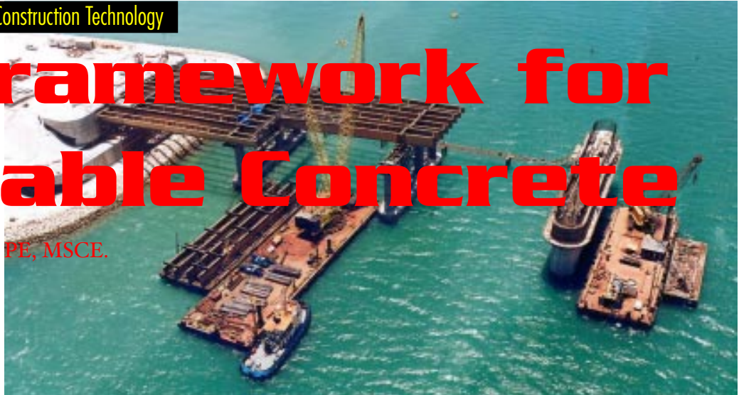
A marine bridge under construction in Bahrain. Concrete elements at this stage were cast using normal practices and were virtually crack-free. Photo courtesy the Ministry of Works and Housing, Bahrain, 2002.
