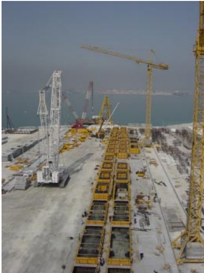
Concrete works at the Port in Bahrain during 2003. Concrete work of the 2.4 km Quay Wall was completed ahead of schedule, with virtually crack-free concrete elements. Photo courtesy of Posford Haskoning Consultants (UK/ Bahrain).
