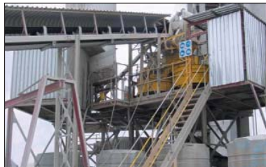
Surface batching plant.
